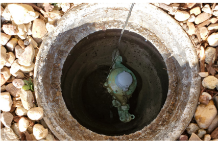
Photo of a water meter that is located in a pit in the front yard.
