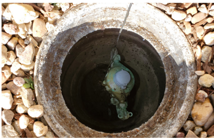
Photo of a water meter that is located in a pit in the front yard.
