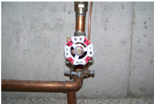
Master shutoff valves are typically located close to where water pipes enter the home. This is often near entryways, but may also be in basements.
